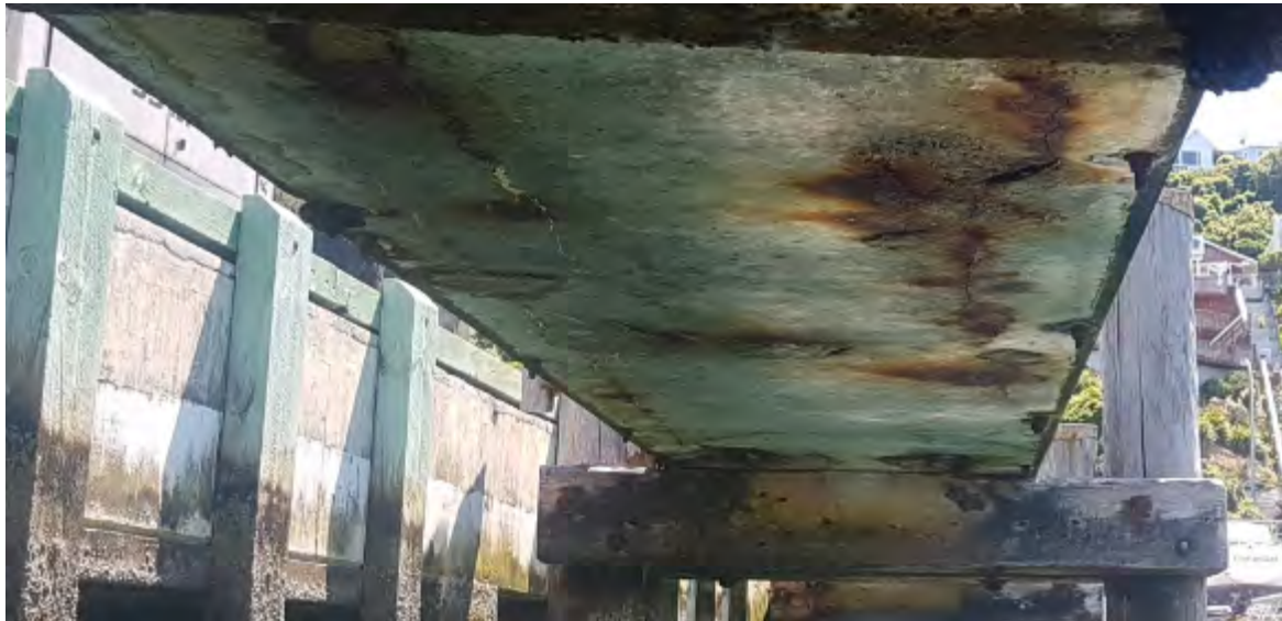
Figure 6-7. Evans Bay Yacht Club South Jetty - Underside of Decking
