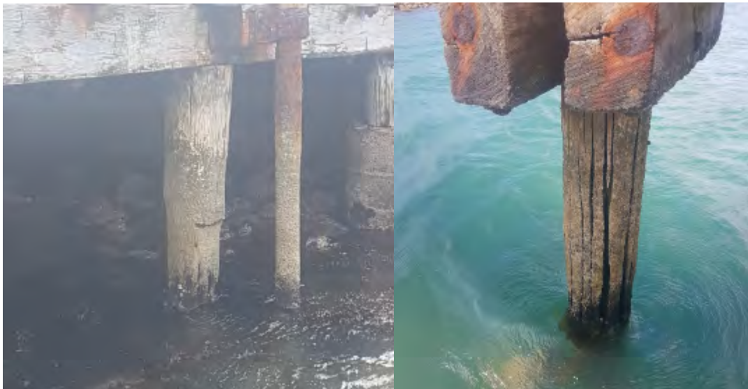
Figure 4-3. Cog Park Jetty, Piles Cross Section Loss and Splitting
