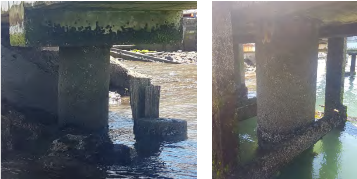
Figure 7-3. Evans Bay Yacht Club Travel Lift – Steel Clad Concrete Piles In Good Condition
