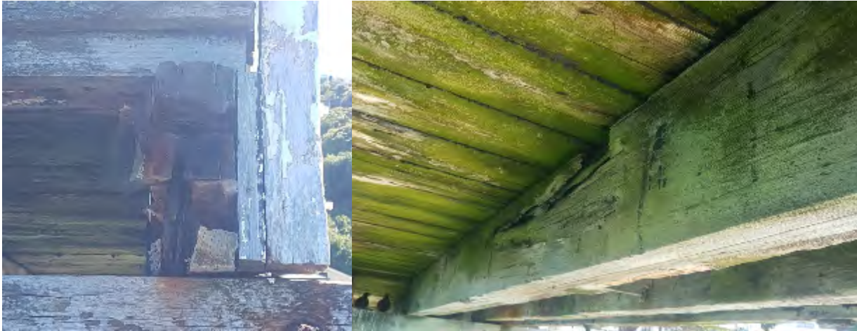
Figure 11-11. Karaka Bay Wharf – Splitting and Cross Section Loss in Existing Joists
