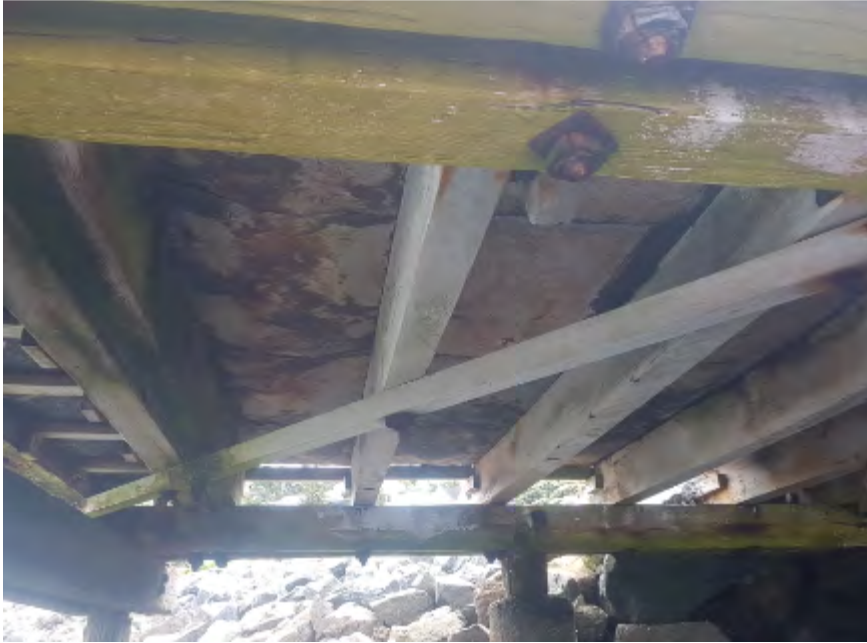
Figure 4-8. Plan Bracing of Decking in a Reasonable Condition
