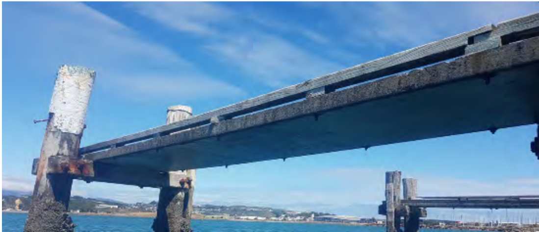
Figure 5-7. Evans Bay Yacht Club Northern Jetty - No Cracking Observed
