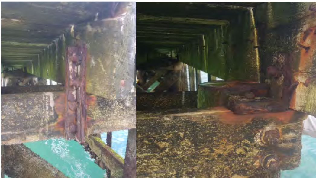
Figure 2-7. Greta Point Wharf – Advanced Corrosion of Bolted Connections
