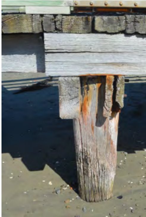
Figure 10-6. Seatoun Wharf – Splitting of Bearer and Joist Ends
