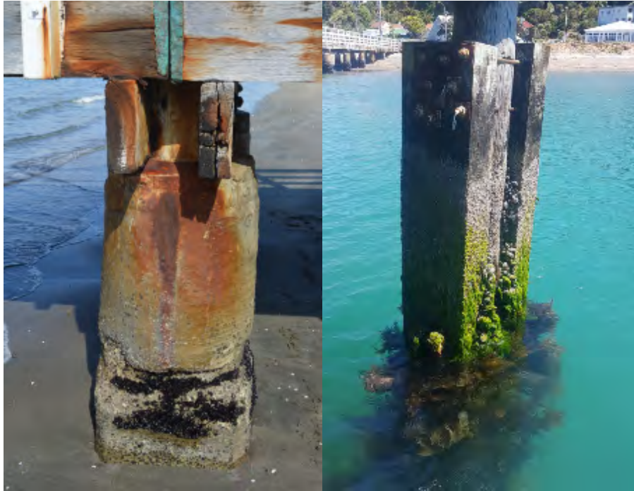
Figure 10-4. Seatoun Wharf – Left, Concrete Encased Timber Piles, Right, Previous Repair of Timber Piles By Sistering
