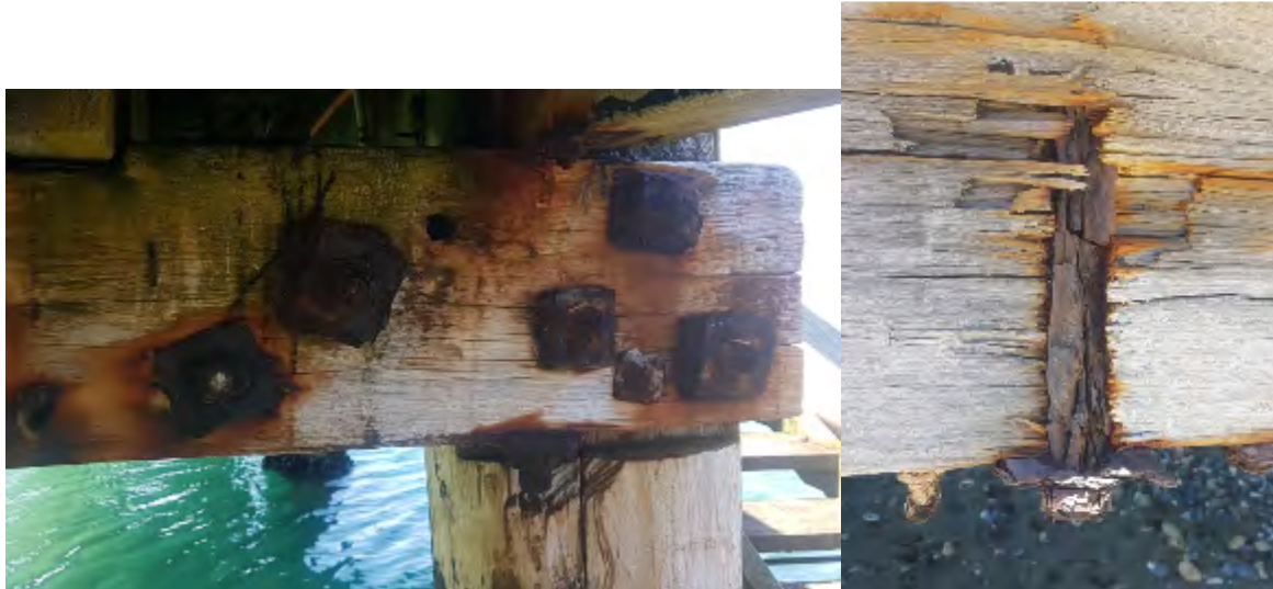
Figure 10-13. Seatoun Wharf, Observed poor condition of bolted connections
