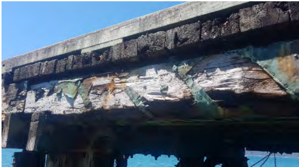
Figure 10-9. Seatoun Wharf – Torn and Missing Copper Cladding, and White Rot on External Bearer, C3-C4
