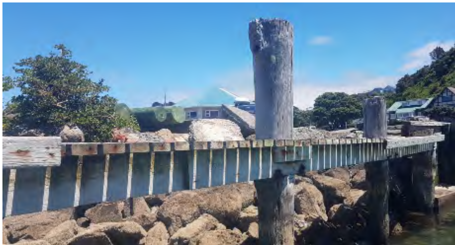
Figure 9-7. Evans Bay Boat Ramp South Jetty – Missing Deck Edging Plank
