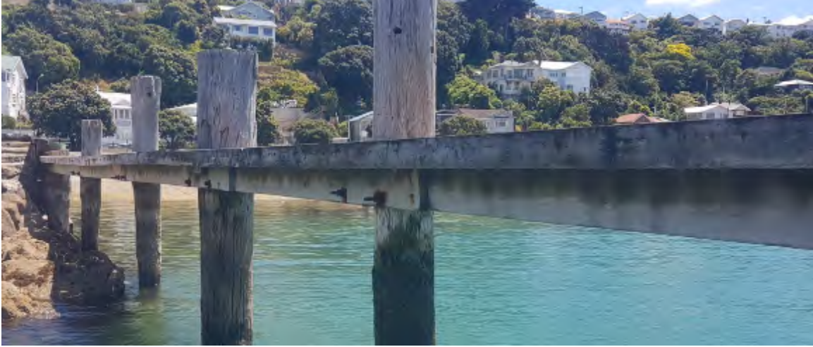
Figure 9-4. Evans Bay Boat Ramp South Jetty – Overlapping of Decking Joists
