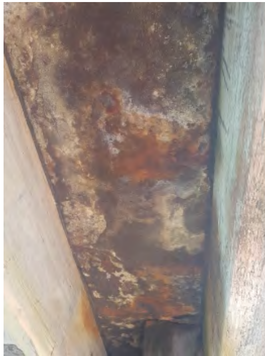
Figure 4-7. Cog Park Jetty - Underside View of Concrete Deck With Advanced Corrosion of Steel Soffit Formwork
