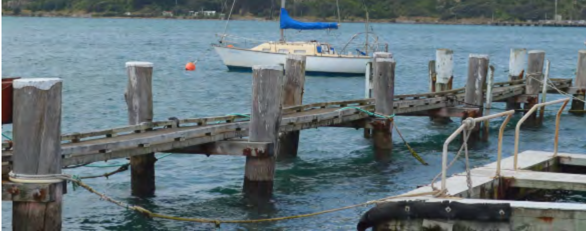
Figure 5-6. Evans Bay Yacht Club Northern Jetty, Sagging of Decking
