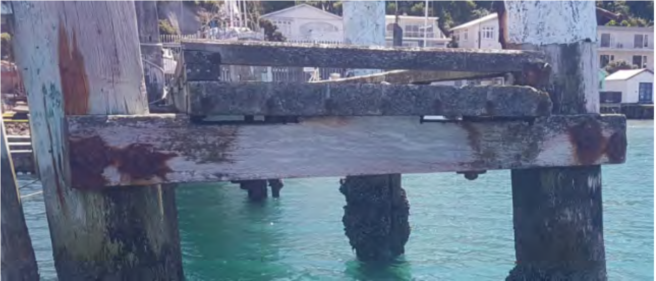
Figure 5-4. Evans Bay Yacht Club Northern Jetty, End Pier Bearer
