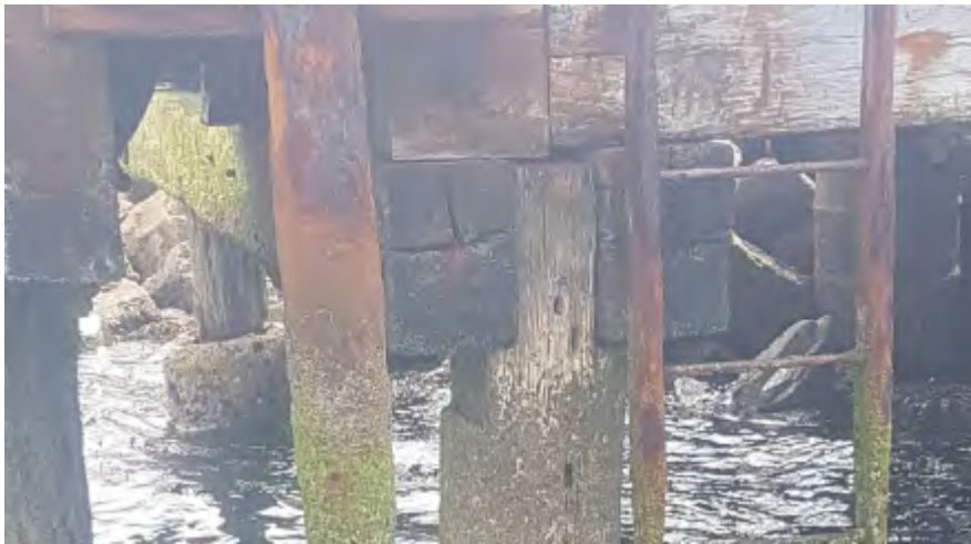
Figure 4-5. Cog Park Jetty – Observed Splitting of Ends of Bearers
