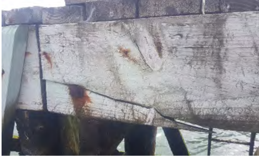
Figure 2-4. Greta Point Wharf - Splitting of Joist
