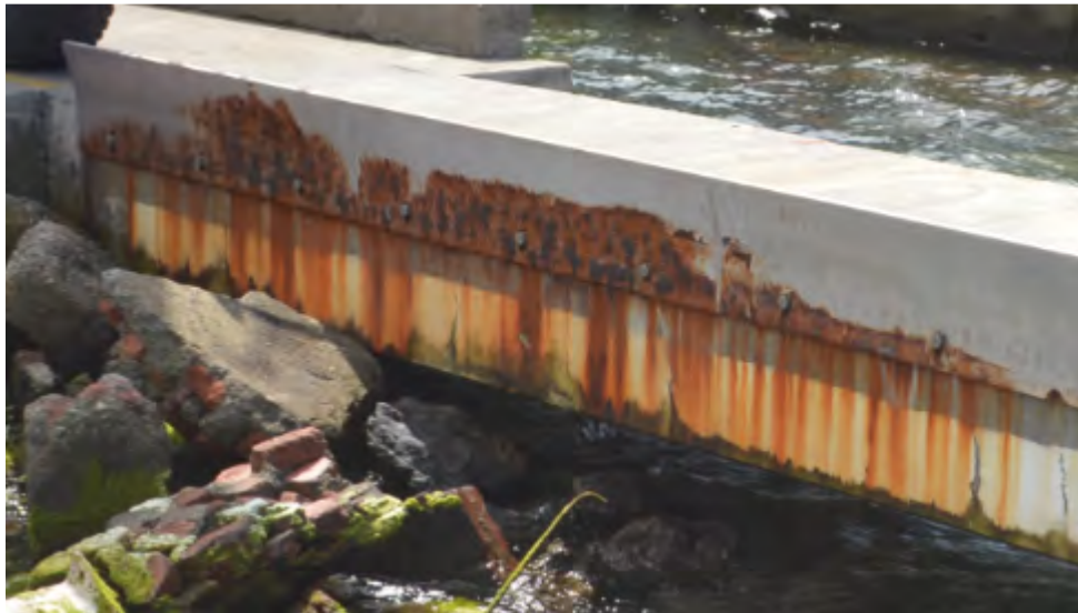
Figure 7-5. Evans Bay Yacht Club travel lift, localised corrosion and rust staining of side mounted steel planks
