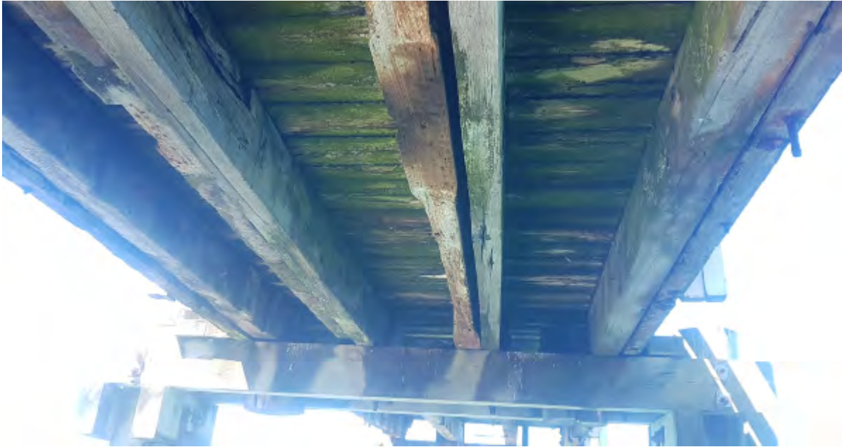
Figure 11-9. Karaka Bay Wharf – Sistered Joists on Intermediate Spans
