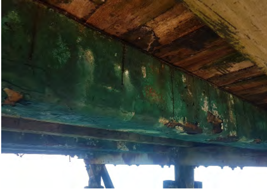
Figure 10-8. Seatoun Wharf – Copper Cladding on Joist
