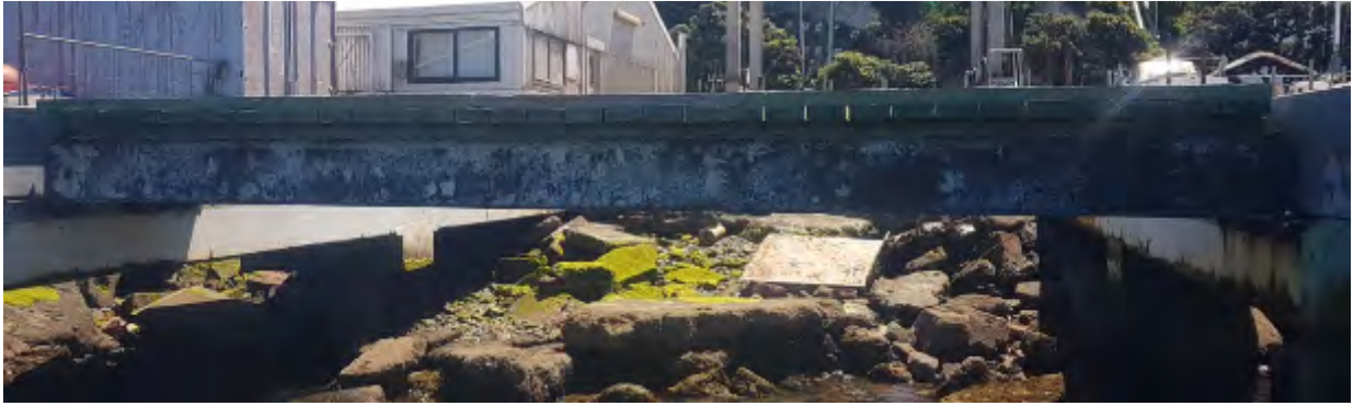
Figure 7-6. Evans Bay Yacht Club Travel Lift - Traverse Access Platform, Steel Beams, Degradation of Paint System
