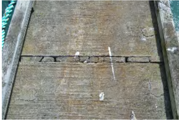
Figure 5-8. Evans Bay Yacht Club Northern Jetty - Cracking of Concrete Decking Stitches
