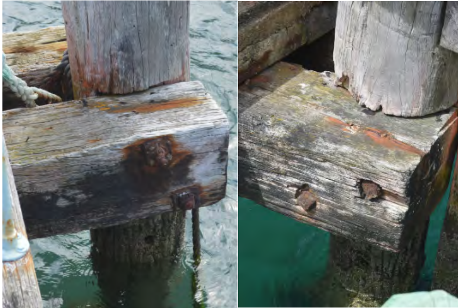
Figure 6-8. Evans Bay Yacht Club South Jetty - Advanced Corrosion of Bolted Connections
