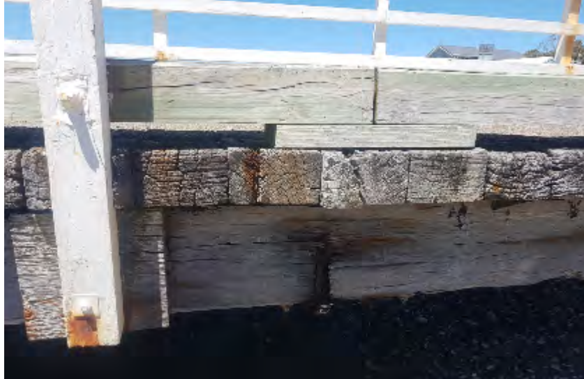
Figure 10-10. Seatoun Wharf – End Splitting of Decking Planks
