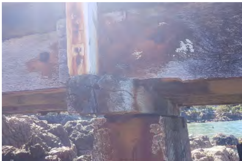
Figure 11-8. Karaka Bay Wharf – Bearer End Splitting and Onset of White Rot
