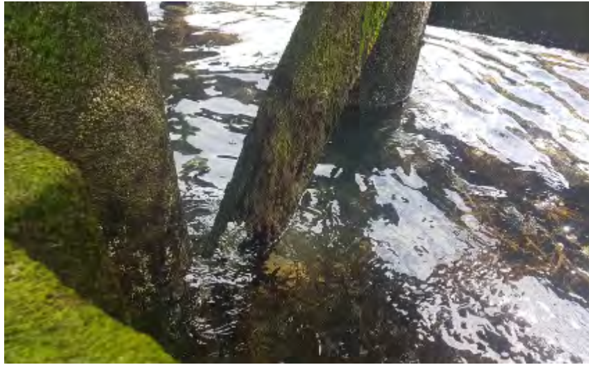
Figure 2-6. Greta Point Wharf – Deteriorated Pile Bracing
