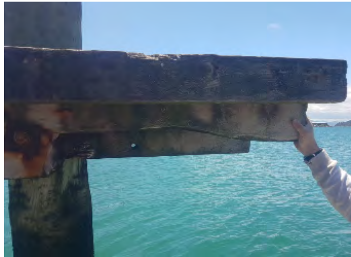
Figure 9-5. Evans Bay Boat Ramp South Jetty – Joist Split With Broken Off Timber Section
