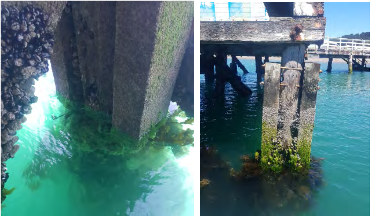
Figure 10-5. Seatoun Wharf - Left, Sistering of Existing Timber Piles Not Fully Extending to Marine Bed. Right, Lateral Shunting of Sistered Piles
