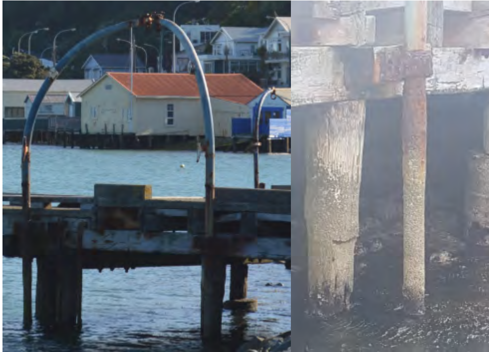
Figure 4-12. Cog Park Jetty - Derek Hoists
