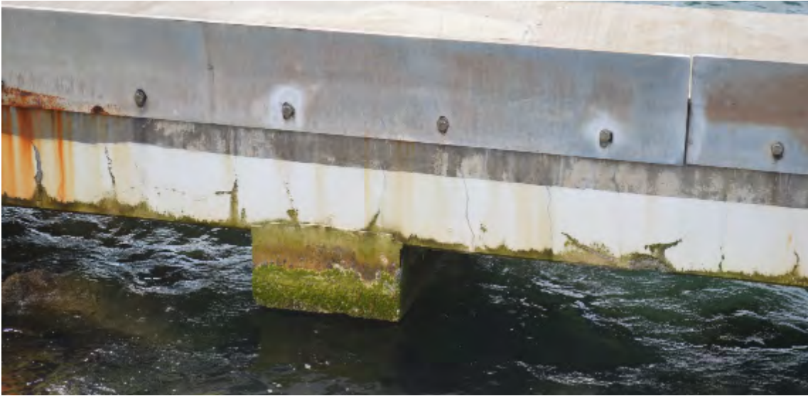
Figure 7-4. Evans Bay Yacht Club Travel Lift - Vertical Cracking on Inside Face of Northern Platform
