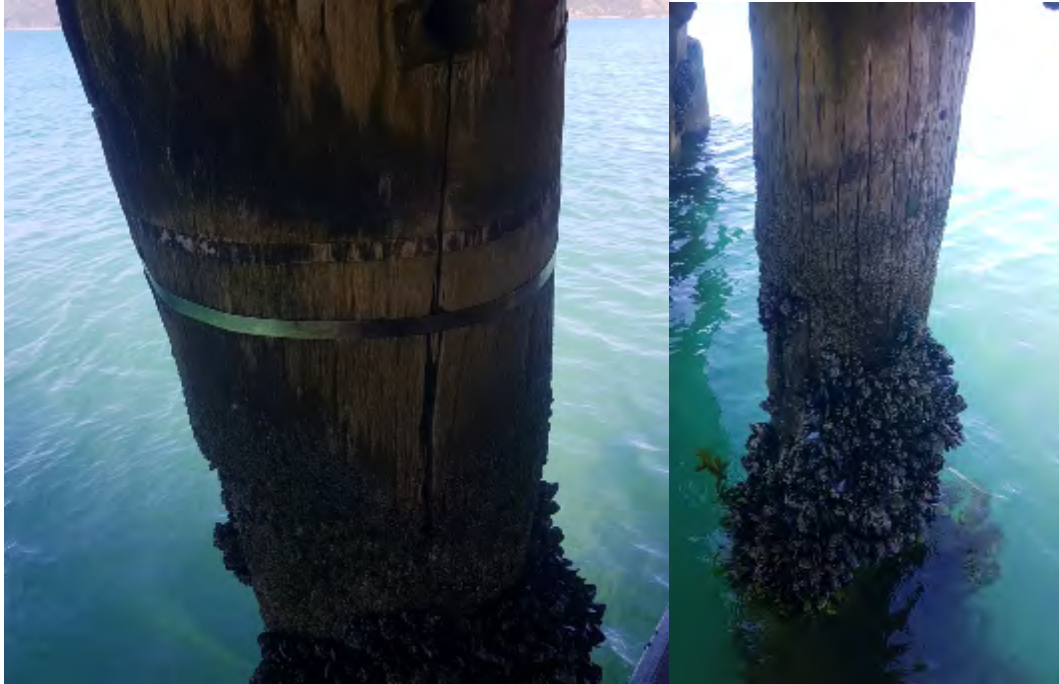
Figure 10-3. Seatoun Wharf - Splitting and Cross Section Loss of Non-Encased Timber Piles
