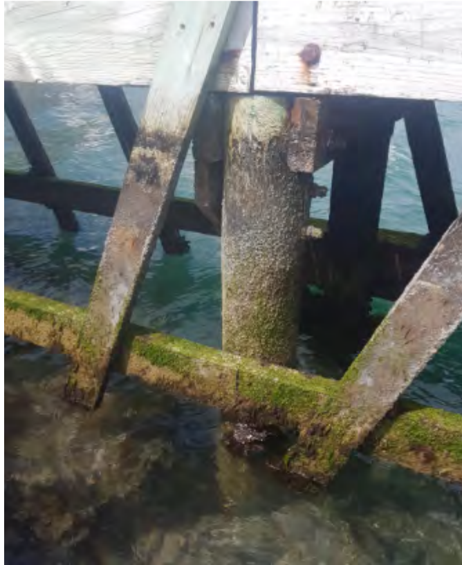
Figure 2-3. Greta Point Wharf - Typical Condition of Piles
