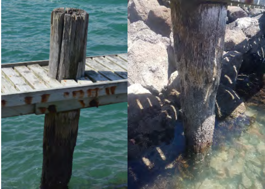
Figure 9-3. Evans Bay Boat Ramp South Jetty - Loss of Cross Section and Splitting of Timber Piles
