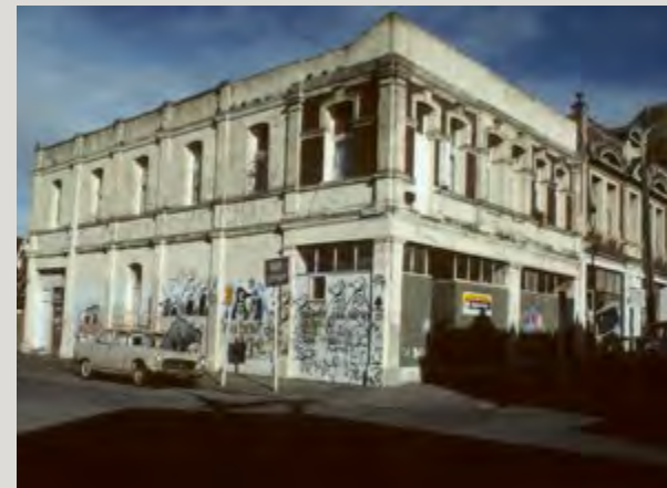
Thistle Hall on Cuba Street was in a poor state of repair in this photograph from 1986. It has since been repaired and refurbished and is now a vibrant community venue and exhibition space.
